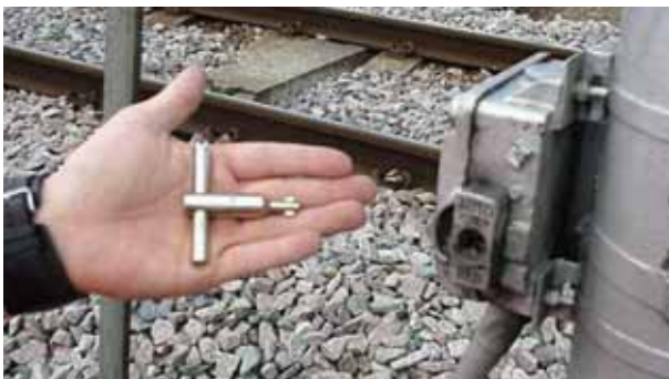
Signal-post replacement key and switch
